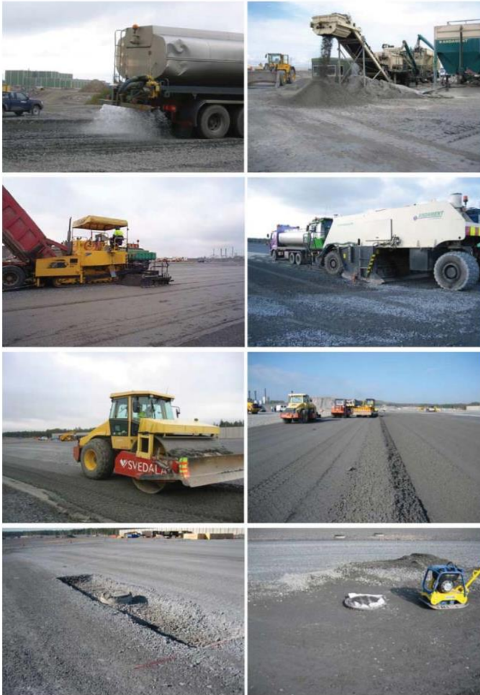
Figure 17. Execution technique. a) Water spraying from a tanker-lorry. b) Mixing of binder-components. c) Laying the mixture by an asphalt paving machine. d) Mixing the crushed rock with the binder-mixture. e) Compaction of the structure with a steel wheel roller. f) Completion of the compacted surface. g) Removal of crushed rock around the wells. h) Filling the excavation around the wells by compacted stabilised mass. [Lahtinen et al. 2007a].
